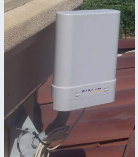
Fig 1.2 Tsunami MP.11 5012 Outdoor Subscriber Unit Mounted on a Rooftop
